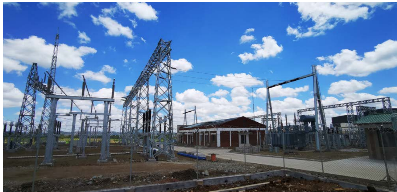
Bikita-Invested 132 kV High-Voltage Transmission Line
