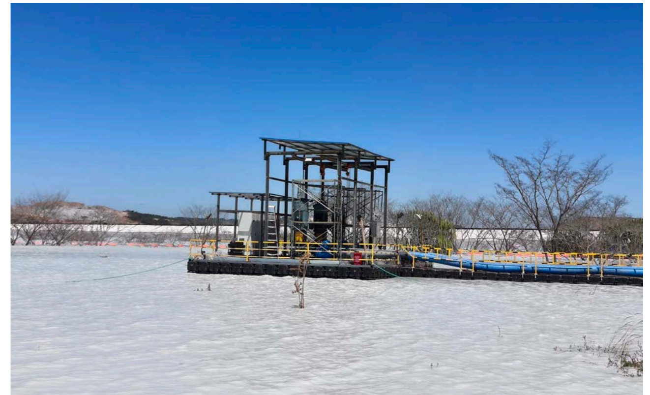
Bikita's Mine Tailings Water Recycling Facility
