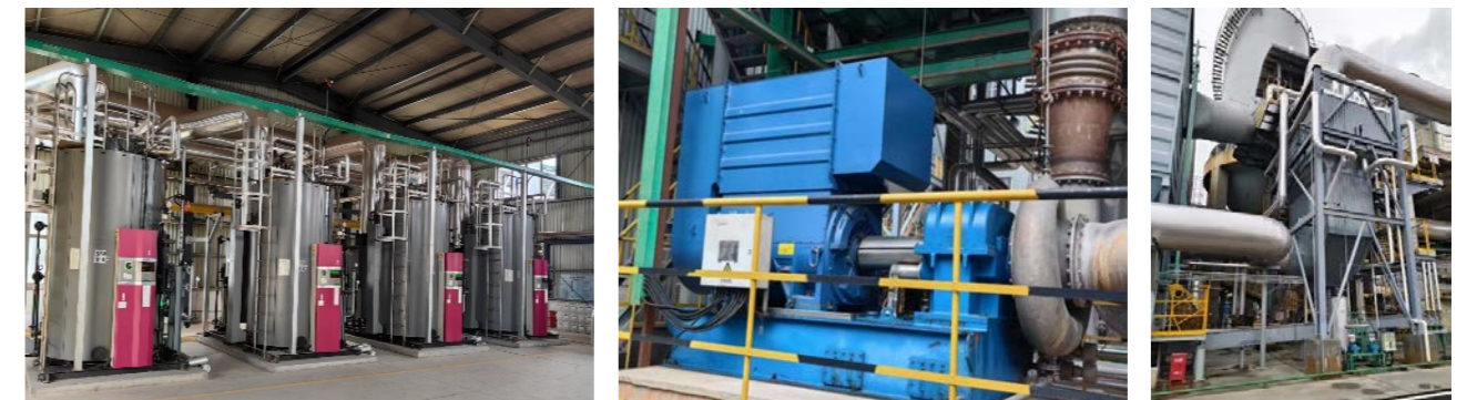
Jiangxi Base Energy Infrastructure: Equipped with high-efficiency boilers, air compressors, and waste heat boilers
