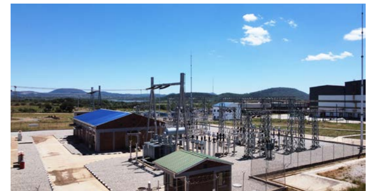
Bikita 132 kV Substation Facility
